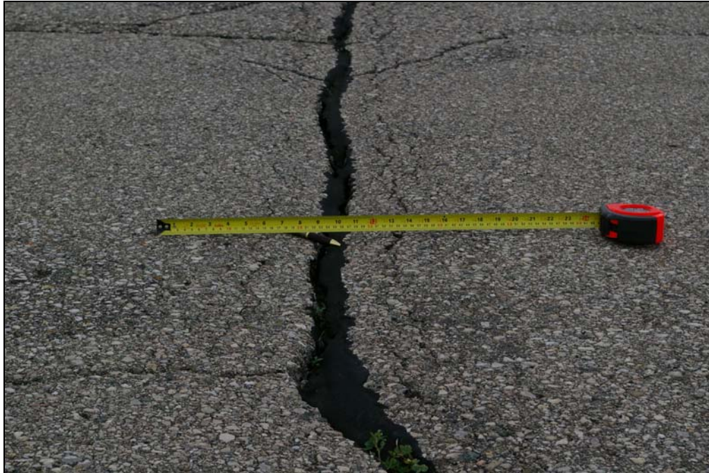
Photo 5: Typical transverse and longitudinal cracks on reconstructed portion of Runway 05-23. Note cupping and secondary cracking at cracks.
