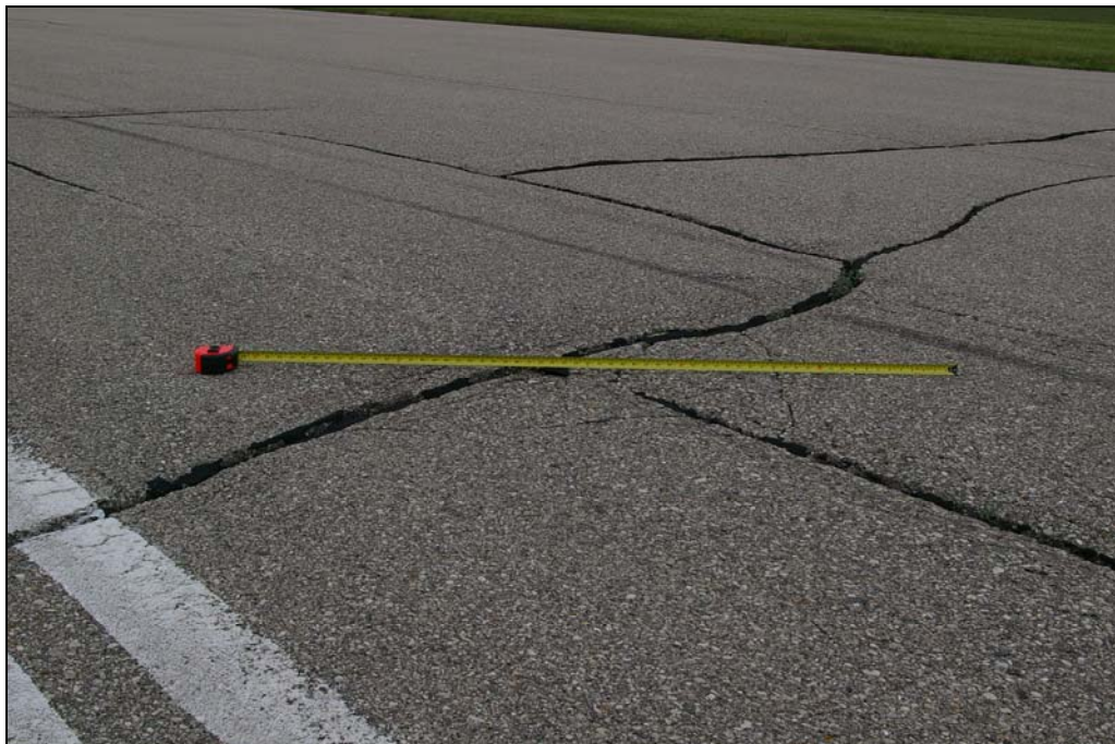
Photo 4: Typical transverse and longitudinal cracks on reconstructed portion of Runway 05-23. Note cupping at cracks.
