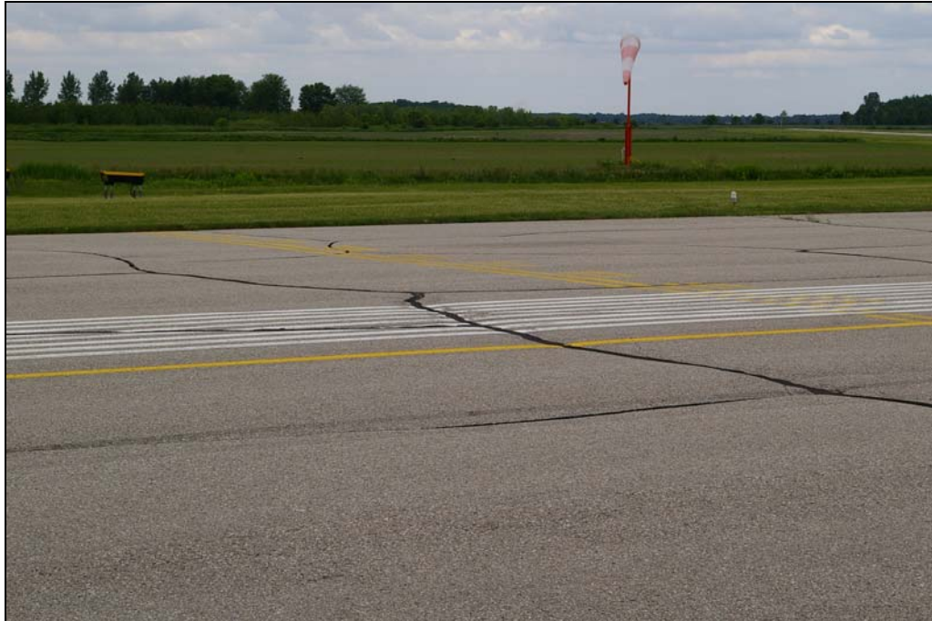
Photo 3: Typical transverse and longitudinal cracks on reconstructed portion of Runway 05-23. Note cupping at cracks.
