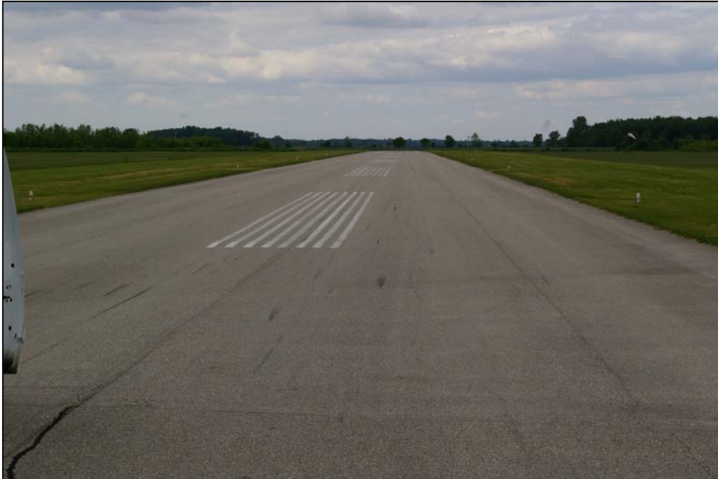
Photo 10: Typical condition of northern portion of Runway 17-35 (1995 construction).
